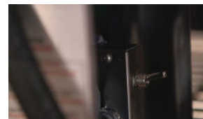
Filter Pump Switch
