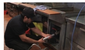
Fryer Drain Pipe
